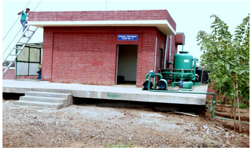
SEWAGE WATER TREATMENT PLANT - 1
